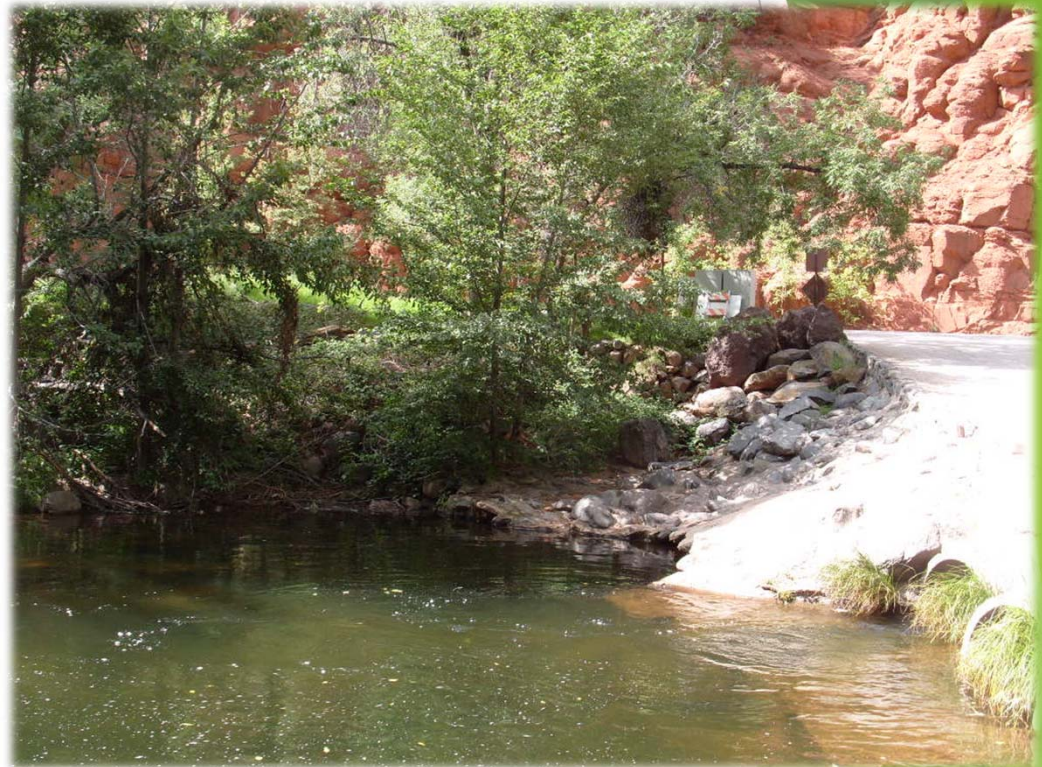
A view of the downstream apron and bank erosion
